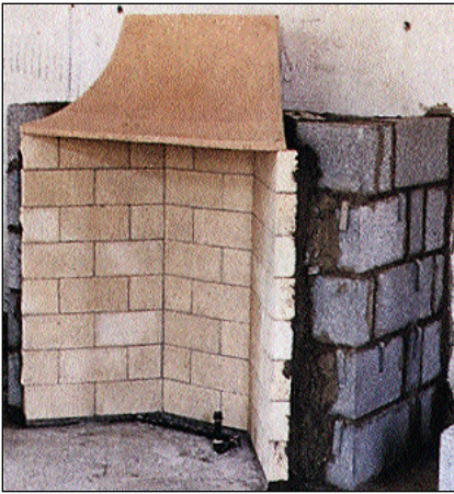
Build the Rumford firebox with 9-inch standard firebrick; then set the curved Rumford throat in the refractory mortar on top of the firebox.
